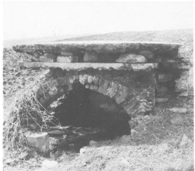
The Intake House as it was in April 1979 showing the degree of vandalism which has occurred. Since then it has been almost totally destroyed.
